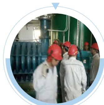
电厂脱硫 Power Plant Desulfurization
