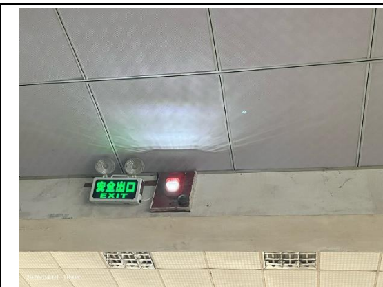
Fire alarm testing
