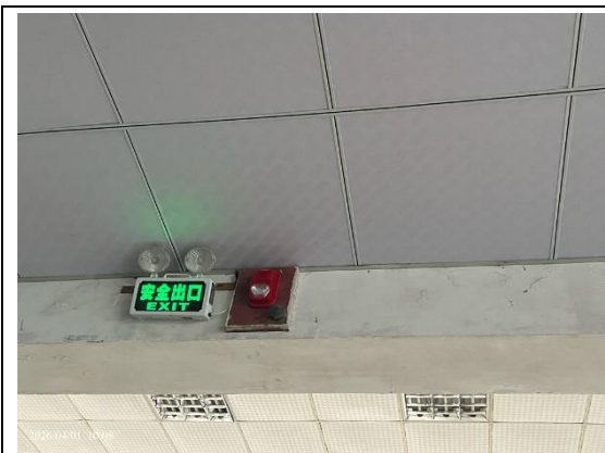
Fire exit sign & Emergency light
