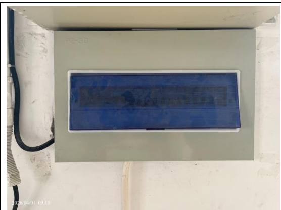
NC-7.9 No warning sign was posted for sampled electricity switch boxes.
