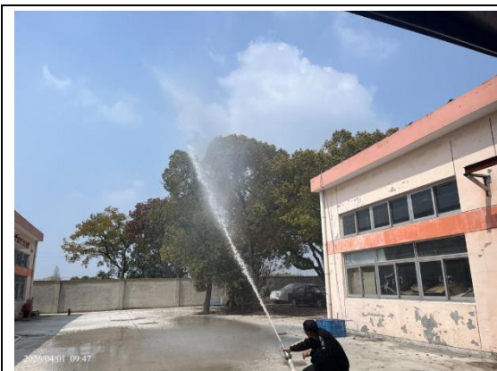
Fire hydrant testing
