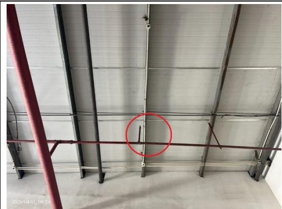
Sprinkler system & smoke detector
