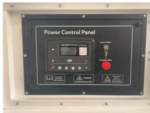
DSE7320 Control Panel NFPA 110 Lvl 1 | Auto-Start Ready
