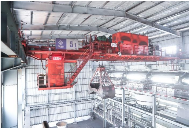
韶关钢铁 无人化抓斗起重机 Shaoguan Iron and Steel Unmanned Grab Crane
